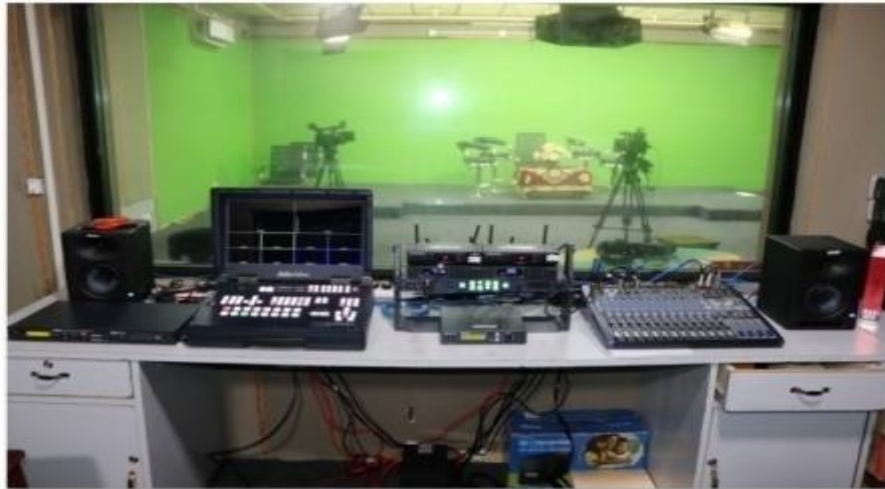
PRODUCTION CONTROL ROOM (PCR) EQUIPPED WITH HS 1300 DATA VIDEO SWITCHER
